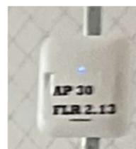
Close up of AP Box
